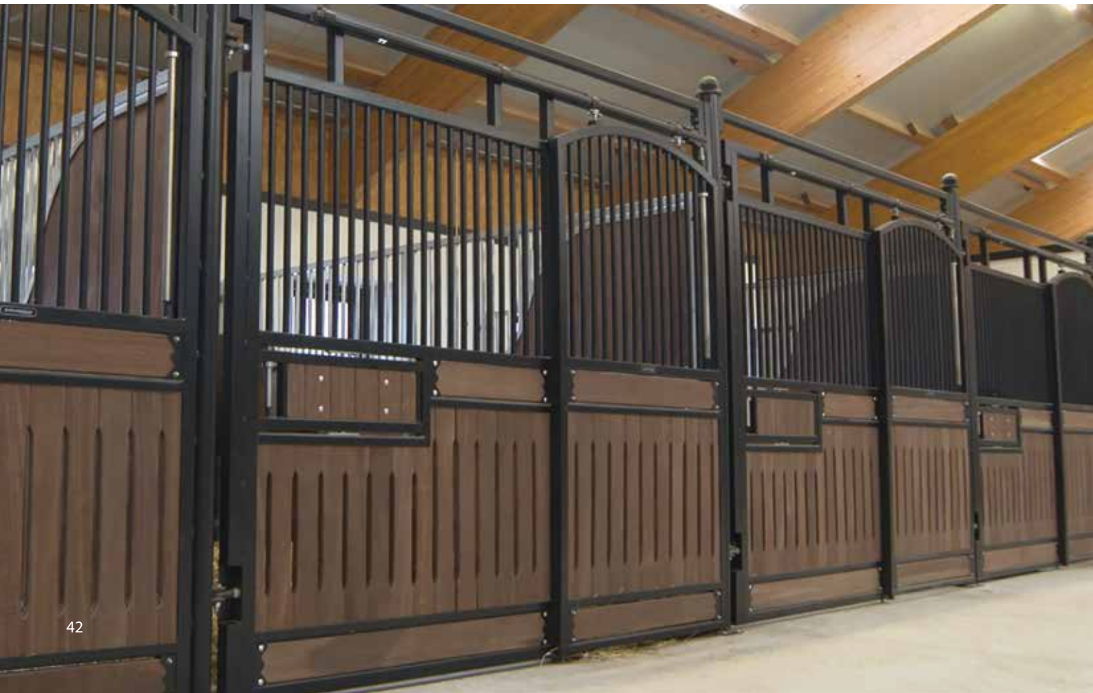
Image below: Nando powder-coated front wall with rotary trough fixture, Ekki wooden panelling with vent slots
